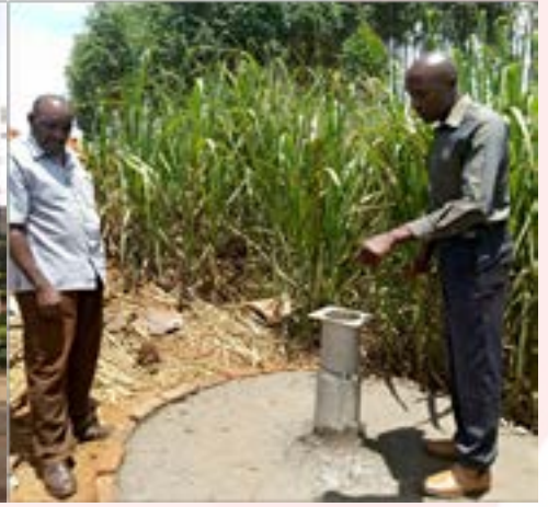
Eng. Mwembe and the chairperson LCIII, Kakira TC while checking on the progress of the borehole construction at Kagoma gate
